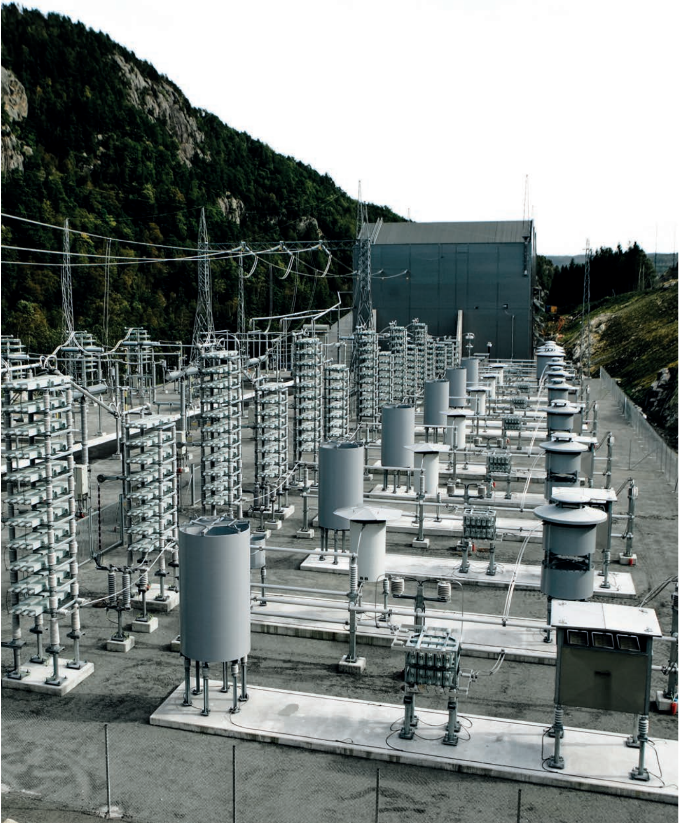
Compensation facility. Photo: Erik Thollaug, Statnett
